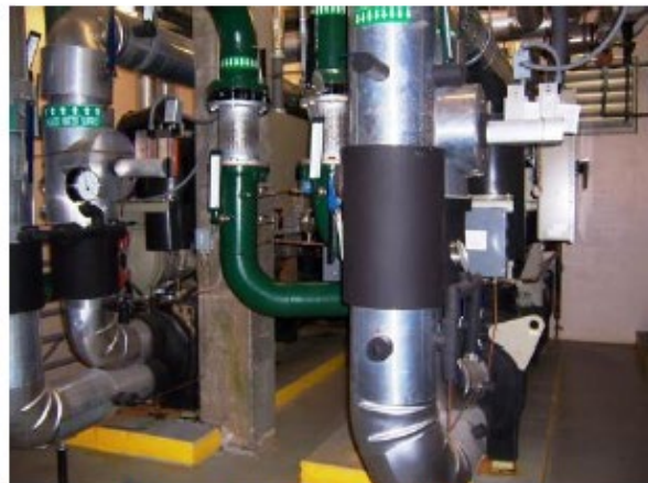
Interior room of chiller room
